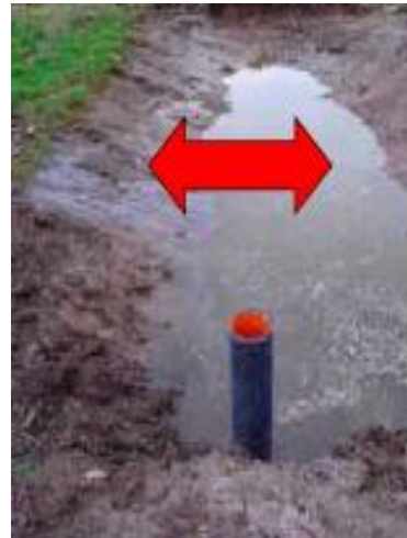
4. Rotate right angle to control water flow. Currently in upright position, retaining water flowing in to scrape from upstream sub surface drainage pipe
